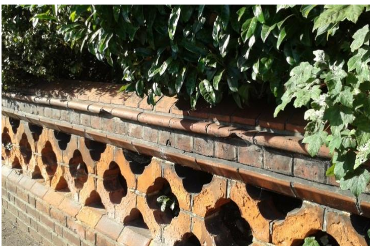
Traditional walls at risk
