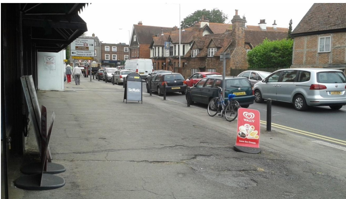
Trip hazards – poorly maintained pavement surface on north side of Church Street (technically outside CA)
